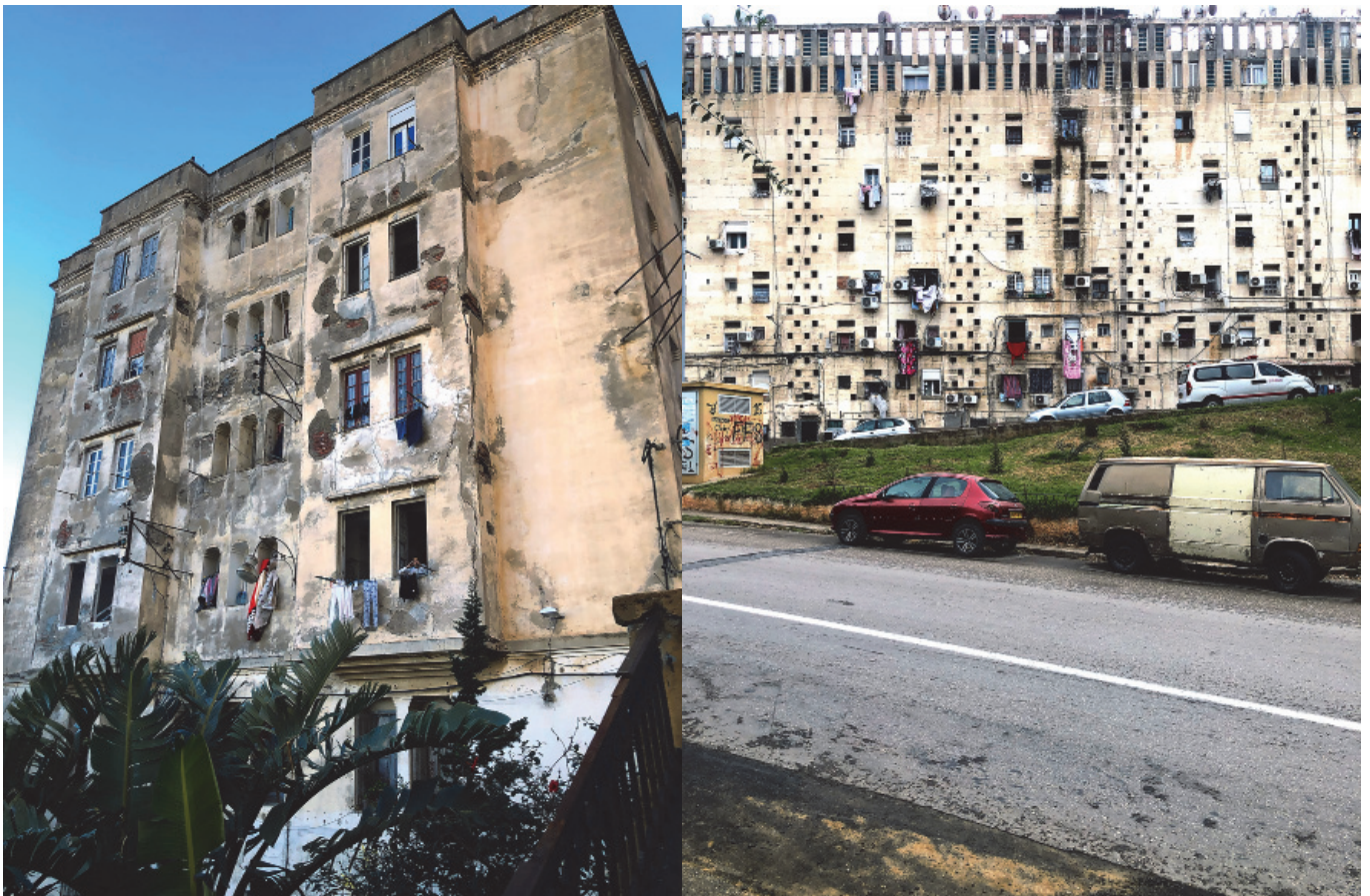
Residential buildings: Boulevard Verdun and Climat de France, Algiers, 2023. (Photos: Sebastian Anderson)
